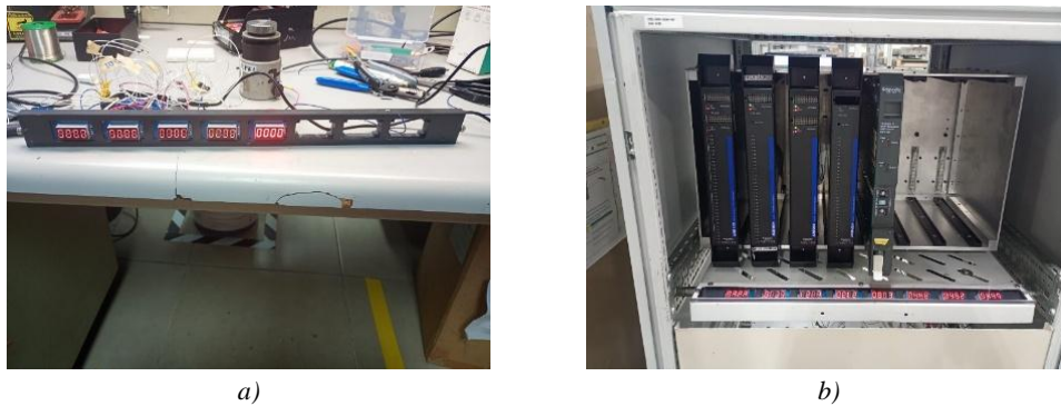
Figure V. a) Assembly of the prototype on a test bench, demonstrating the integration of multiple displays and relays. b) Installation of the prototype in the production line's test cabinet.
