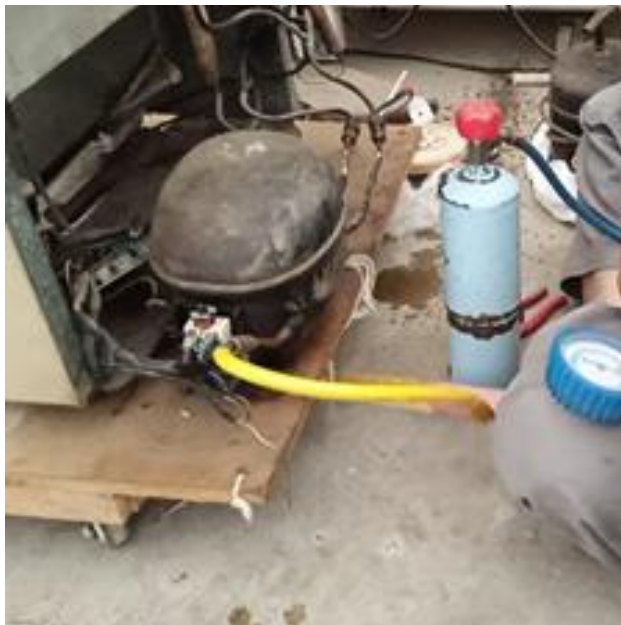
Figure VIII.- Charging R-134a Refrigerant
